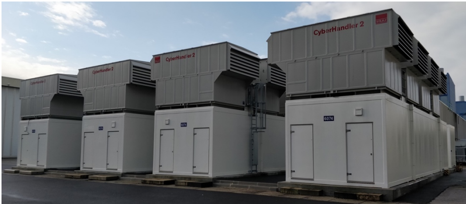
CRO EPN computing center at Point 2
