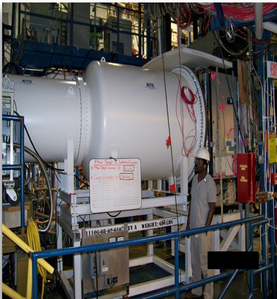
2-stage vacuum box in Hall B beam line
